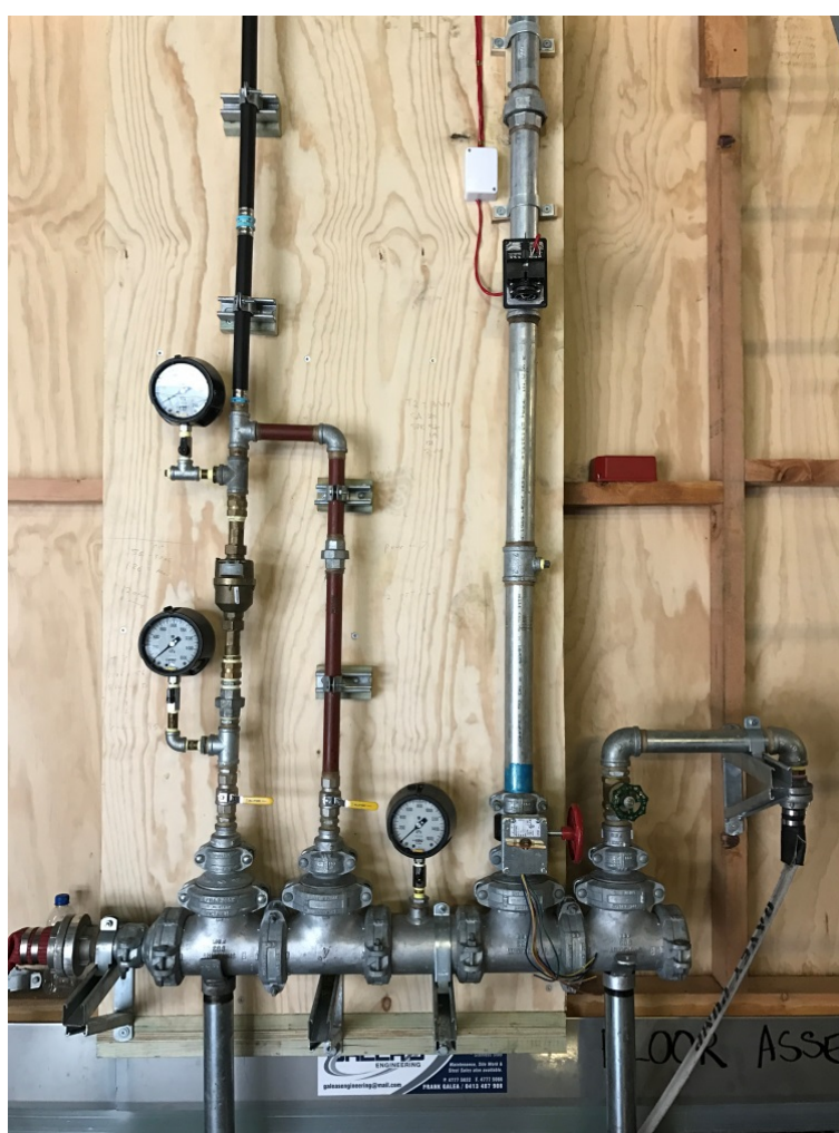
Figure 4 Photo showing the two sprinkler systems. To the left is the 25 mm polyethylene piping of System 1 (Domestic), and to the right is the 50 mm steel piping of System 2 (Hydrant).
